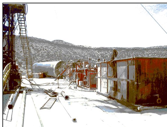
Figure 1. Specialized equipment for well workover, including a water tank, hydraulic power for rotating head, mud pump, and mud pit.
