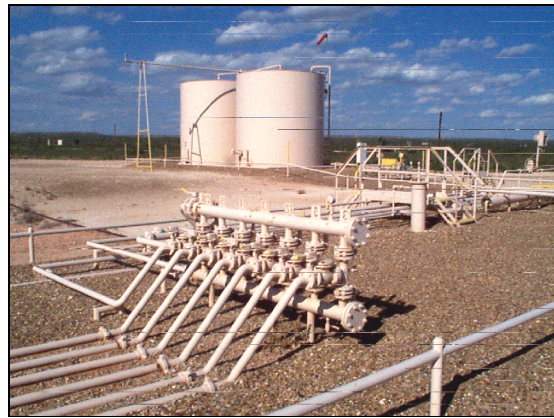
Figure 2. Flow lines entering the header. Often the lines are numbered like these for easy identification.
