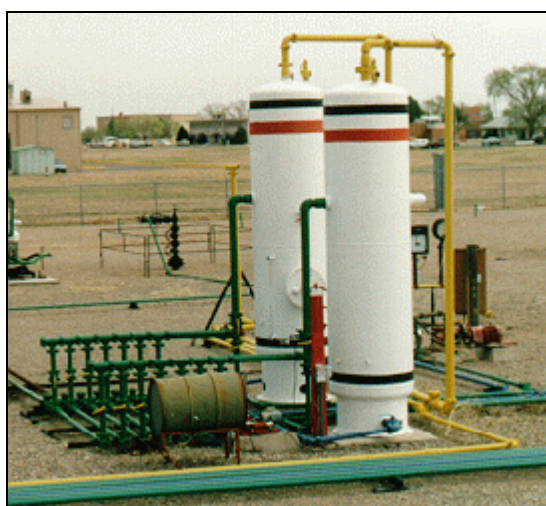
Figure 4. A chemical injection system using a barrel and pump.
