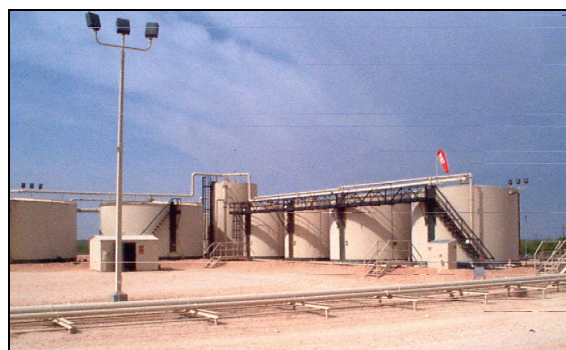
Figure 1. Tank battery atmospheric vessels including a gun barrel, four oil storage tanks, and two water tanks.
