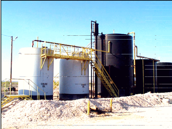
Figure 11. The dike around a tank battery should be able to hold a volume one-and-one-half times the capacity of all of the vessels.
