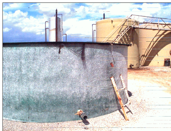
Figure 10. A water disposal tank.
