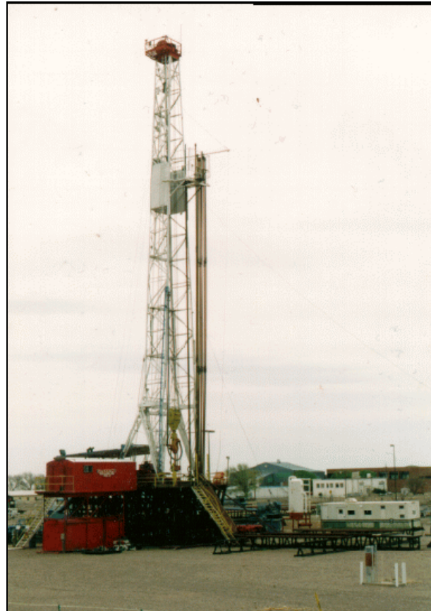
Figure 1. A drilling rig in erected to bore a well. Note the pipe in the rack alongside the derrick.
