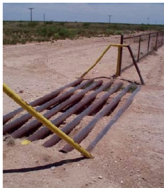
Figure 3. A poorly maintained cattle guard.
