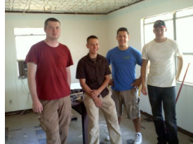
Altus Air Force Airman working on renovations at donated house for transitional living program.
